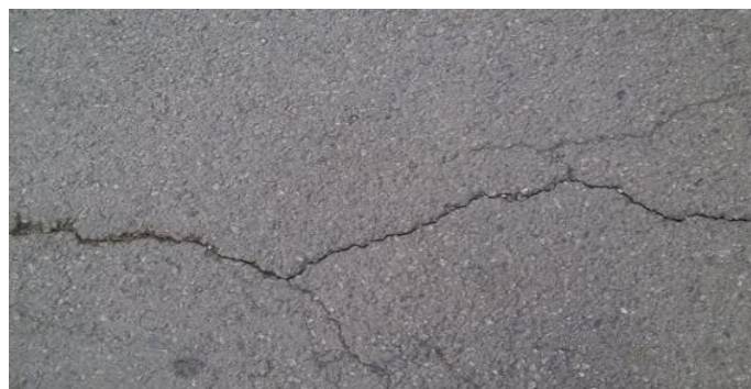
Fig 7. The sample crack image
